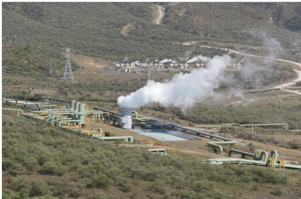
Photo: Geothermal Power Plant of KenGen in Kenya (Source: Runar Magnusson, 2016)
